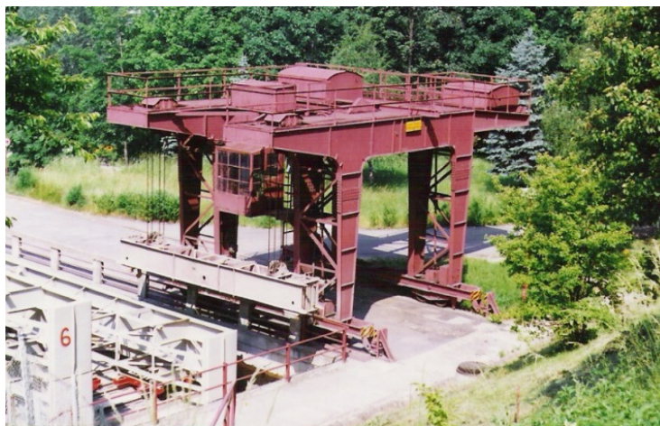
Fig. 3. The view of the portal gantry crane
